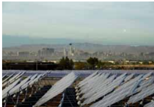
(Pictured left) Nellis AFB photovoltaic solar facility
