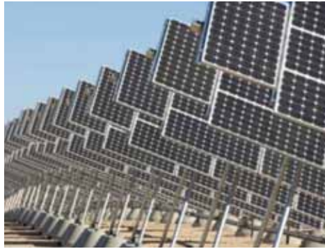
(Pictured right) Nellis AFB photovoltaic solar facility
