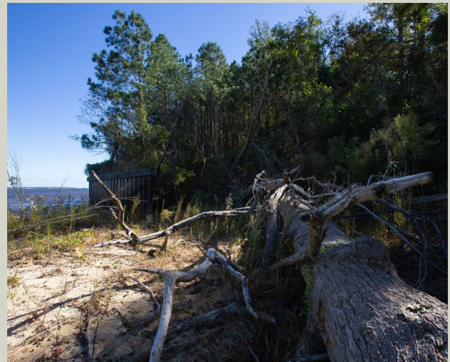
Hurricane Florence, a Category 4 Hurricane, damaged over 5,000 linear feet of shoreline along the Neuse River in 2018. Marine Corps Air Station Cherry Point received $1 million through the 2020 National Coastal Resilience Fund to construct a 1,667 linear foot shoreline near the base along the Neuse River to prevent erosion and mitigate flooding that would damage the installation’s critical infrastructure. (U.S. Marine Corps photo by Cpl. Alexandra Amor Santos Arambulo)
